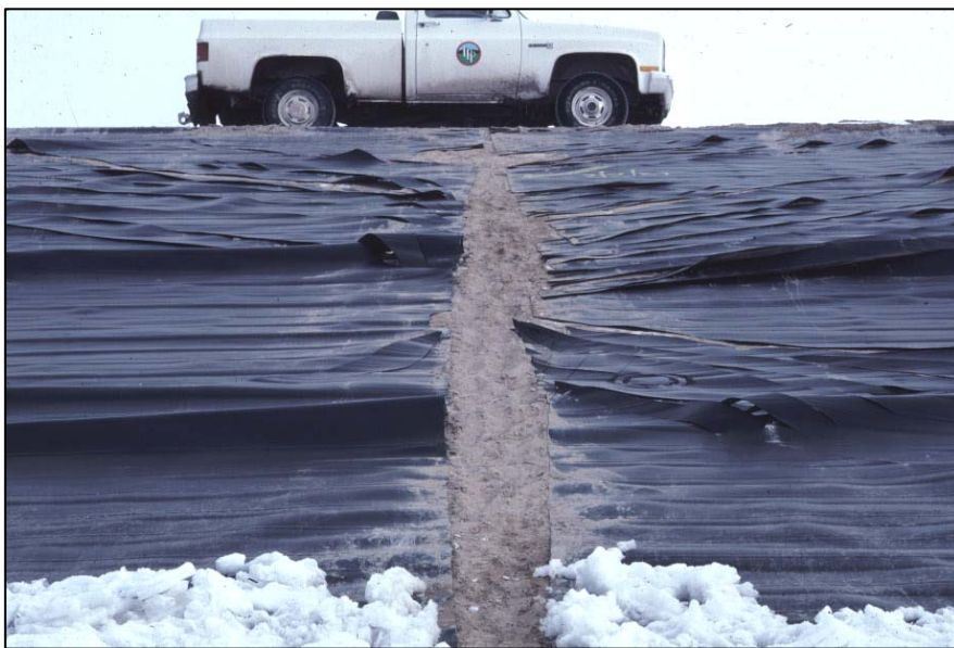
Fig. 1: Cracking of the geomembrane liner observed on the side slope of an empty geomembrane-lined reservoir after an extremely cold night. [Photo J.P. Giroud]
